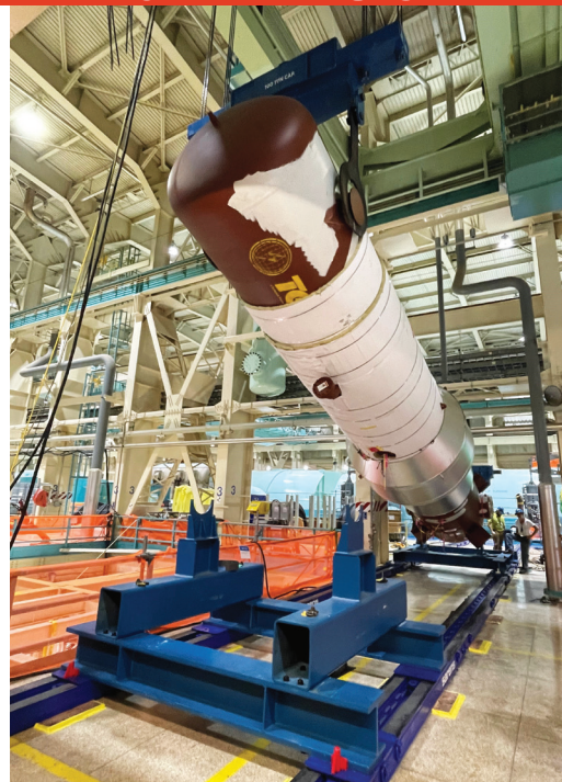
Sarens' involvement on the Oconee Nuclear Station project, lifting two huge feedwater heaters, was completed in just 12 days
