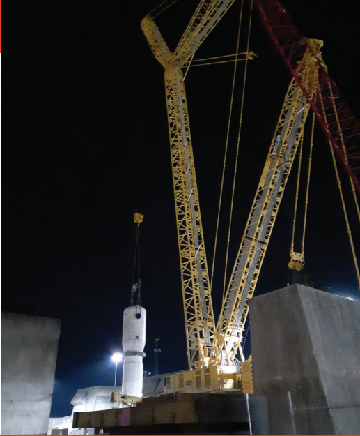
Sarens is involved in many nuclear projects, including the Watts Bar nuclear facility in Tennessee, USA
